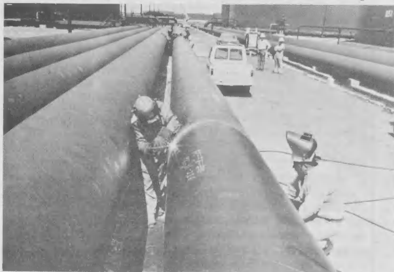
Welders P. Simileer (left) and L. Cuba working on the 36-inch pipeline which is over 5000 ft. long.
